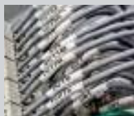
Wire and cable labels
