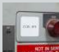
Asset and equipment ID
