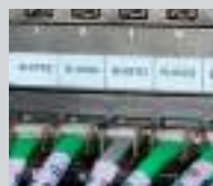
Patch panel and terminal block ID
