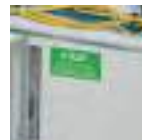
Control panel labeling
